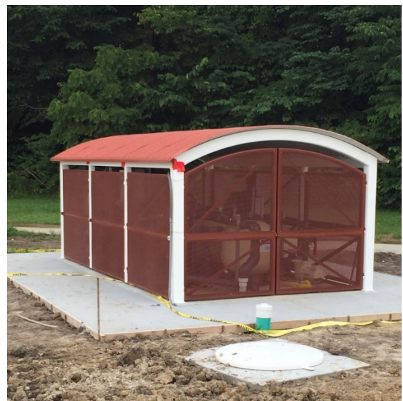
Recirculation mechanicals need to be protected in a small shelter
