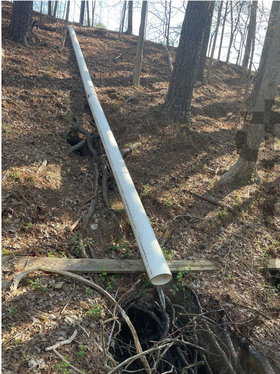
Photograph 6 – Overflow Device Outlet, Erosion Cavity Below Repaired Joint, Erosion Cavity at Outlet
