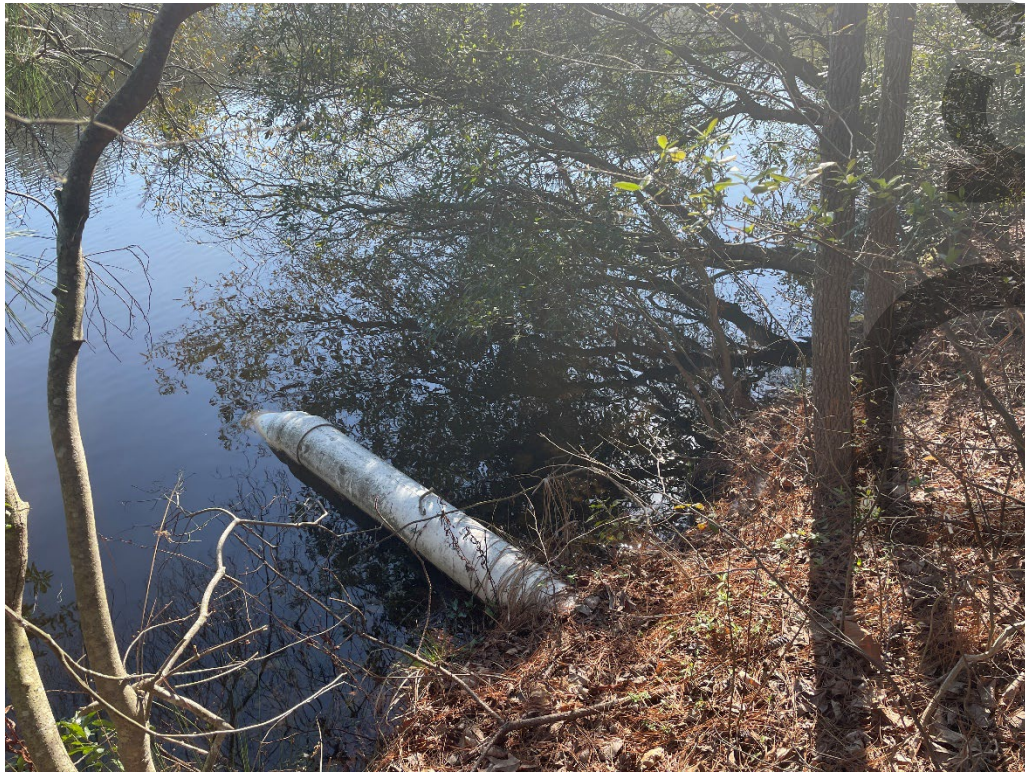
Photograph 4 – PVC Overflow Device Inlet
