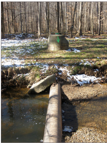
Typical sewer trunk line along Bolin Creek
